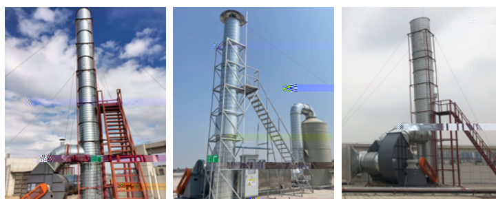
Waste Gas Disposal Facilities
